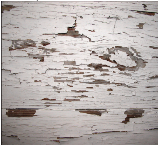
Figure 1. Deteriorated lead-based paint is one of the leading causes of lead poisoning in Detroit children (Photo credit: Emily Wilke).
